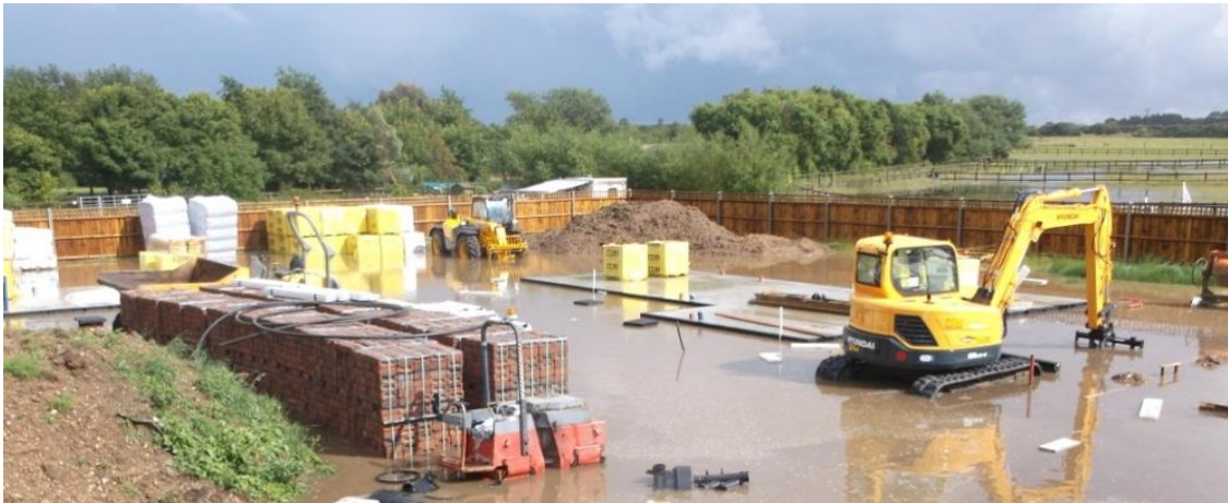
Photo of a development site located on the mapped surface water flood path that flooded in 2016, Hemsby, Norfolk.
