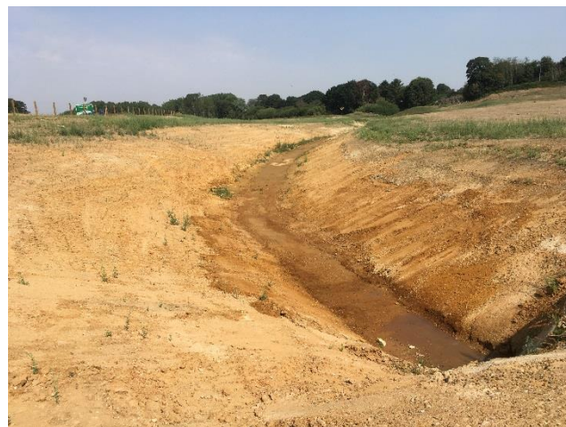
e) Reinstated watercourse and overland flow route (just completed prior to vegetation getting established).
