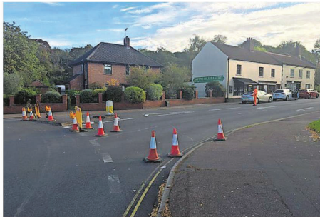
Emergency repairs to a sewer led to the closure of Kett's Hill in Norwich Picture: PETER WALSH.
