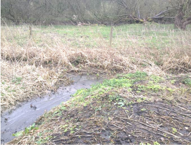
Photo 3.1: Grips directing road runoff to ditch opposite entrance to Weston Hall, with evidence of sediment accumulation in ditch.
