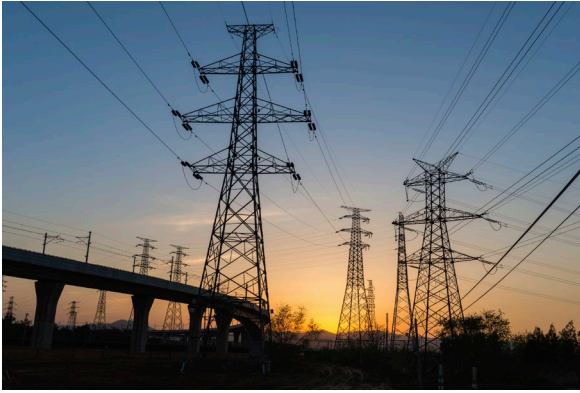
Water and electricity supply is a constraint The Environment Agency and UK Power Networks confirm supply constraints – which will limit housing, commercial and business investment in the county
