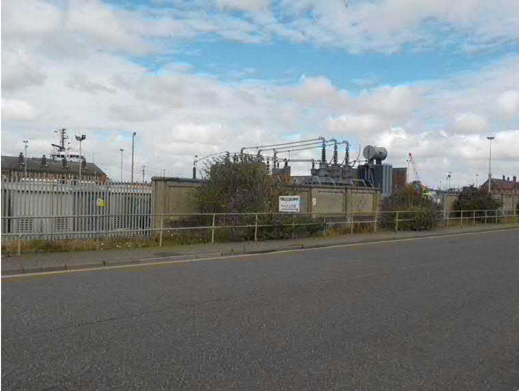
Photograph 3 – Electricity Substation on Southgates Road
