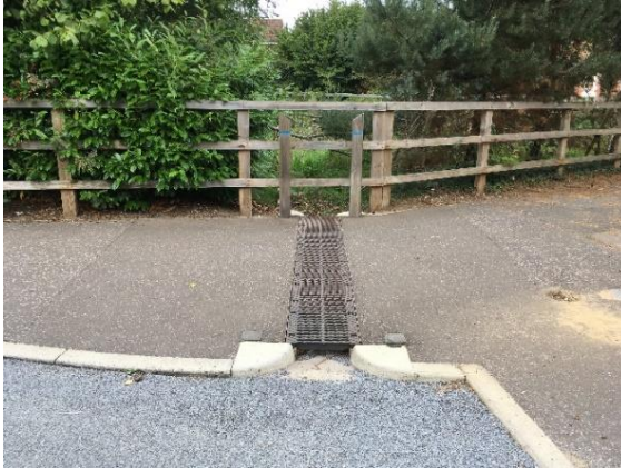
Photo of a rill from a carriageway through a path to a SuDS Basin – Drayton, Norfolk (image E Simpson @ NCC LLFA)
