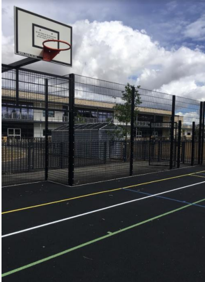
Photo of the use of permeable tarmac on a playground at the SEN School, Old Buckingham, Norfolk (Image E Simpson @ Norfolk LLFA)
