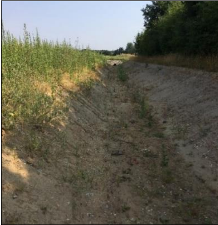
Photo showing a newly created channel as an extension of a watercourse, North Norwich, Norfolk (image E Simpson @ NCC LLFA).
