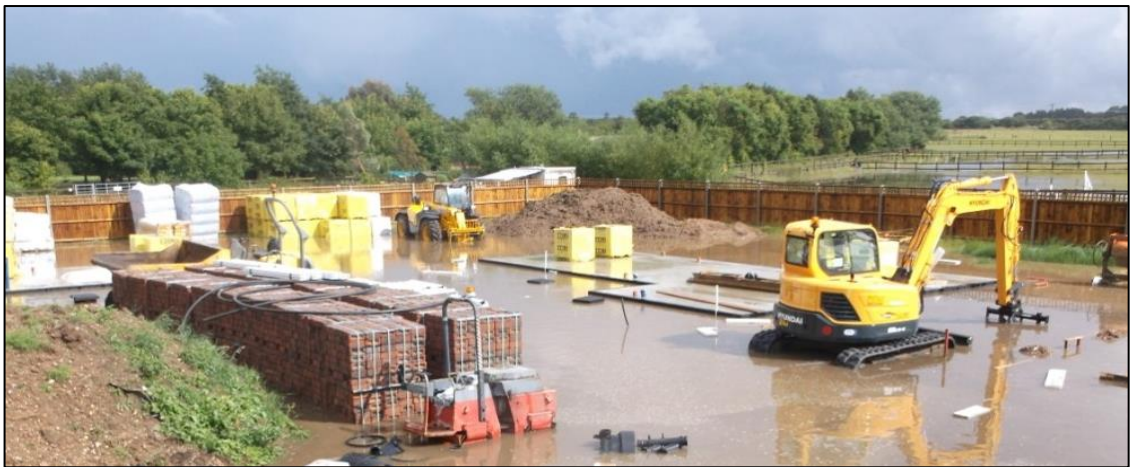
Photo of a development site located on the mapped surface water flood path that flooded in 2016, Hemsby, Norfolk.
